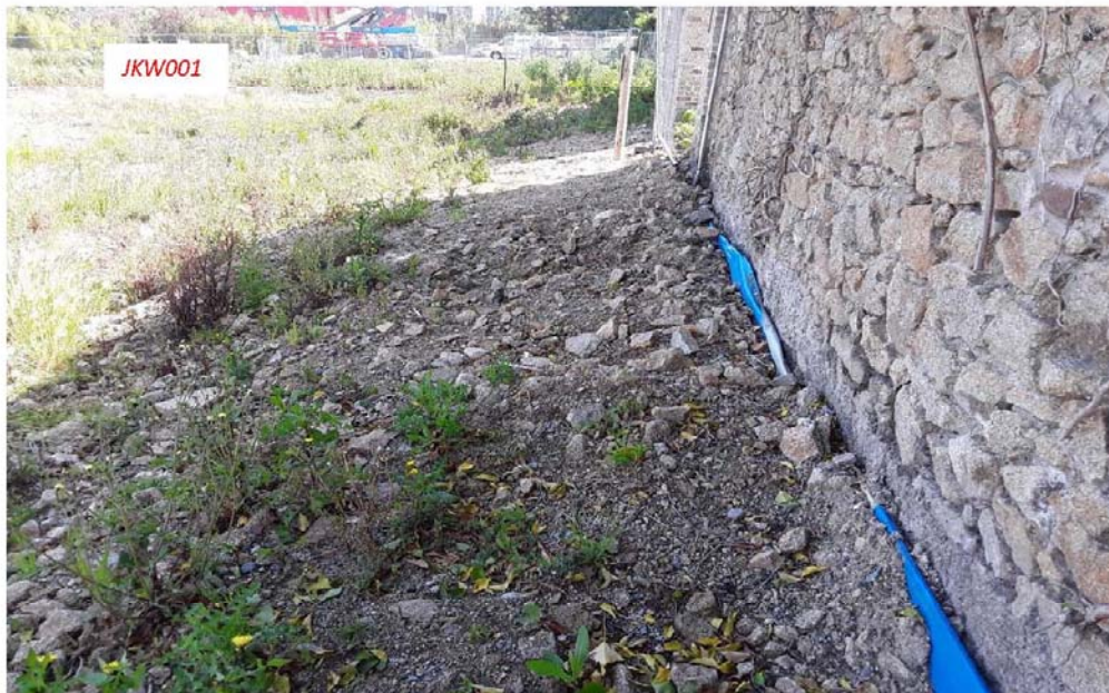
Image of JKW001 from May 2020 inspection. No JKW present.
